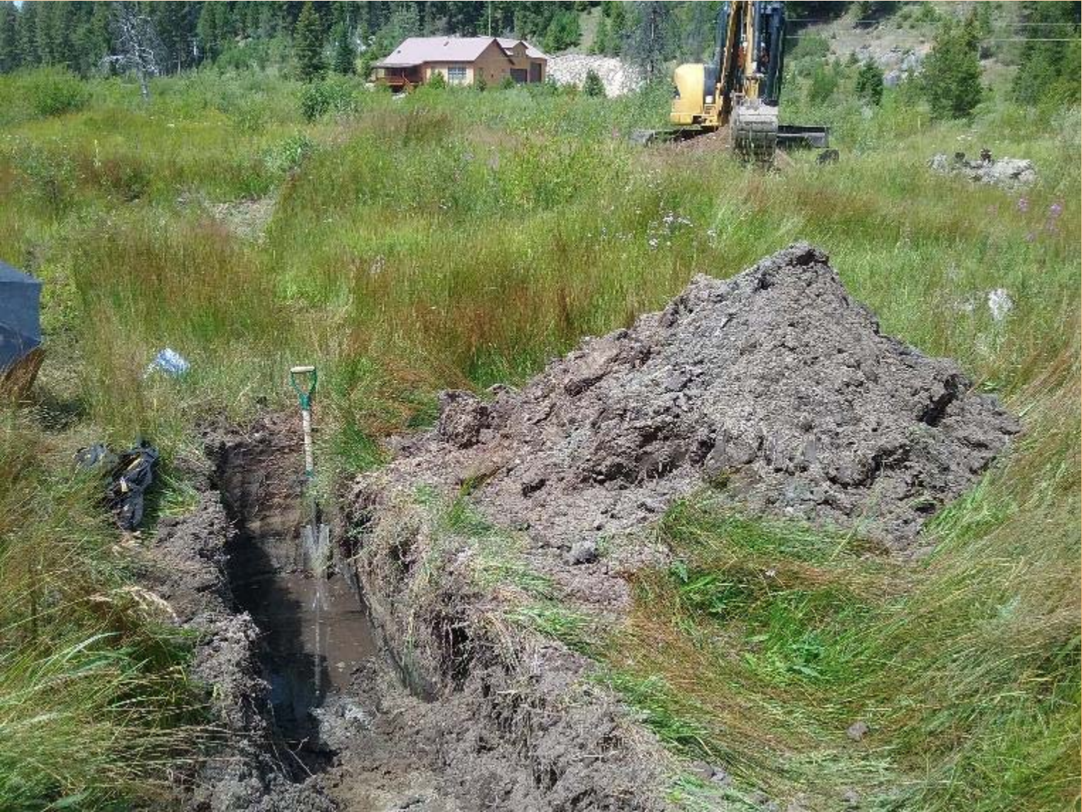
Typical excavator-dug soil pit during the July 23 rd to 26 th 2018 field investigation at Fred Burr Creek.
