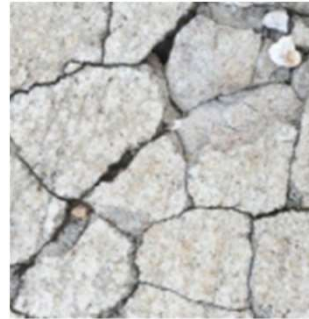
Cracks Form and Leak Methane
